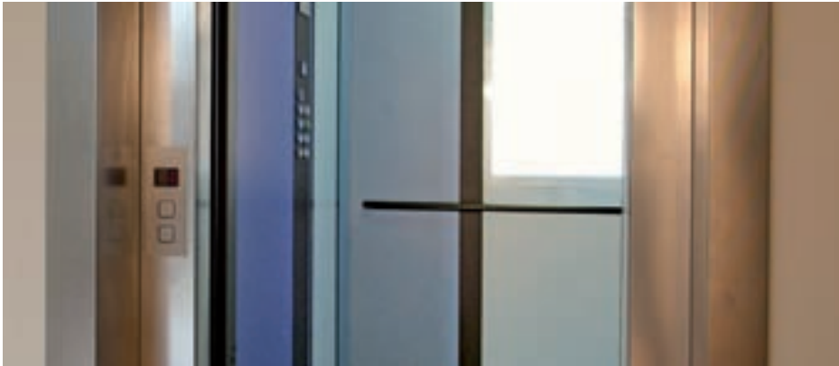
MP PASSENGER lift Don Orione Hospital Milan, Italy.
